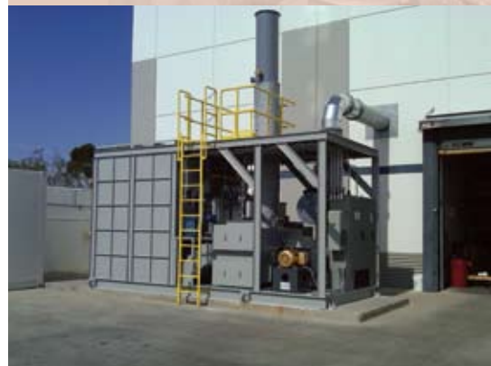
Small regenerative oxidizer installation by Catalytic Combustion Corporation.
