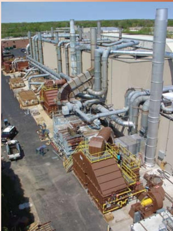
Multiple large Anguil regenerative oxidizers at a manufacturing facility.
