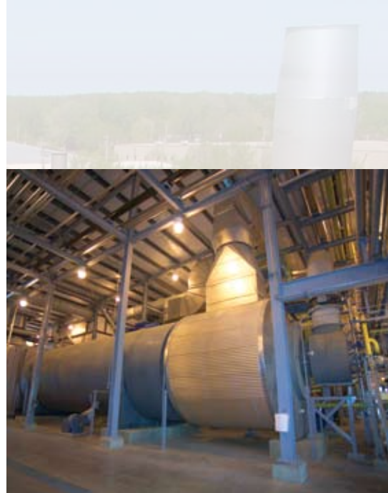
A typical indoor installation of John Zink regenerative thermal oxidizers.
