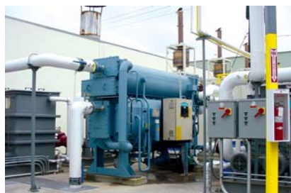
A single-stage steam absorption chiller such as this 160-ton Thermax model can use low-grade waste heat for process or comfort cooling.
