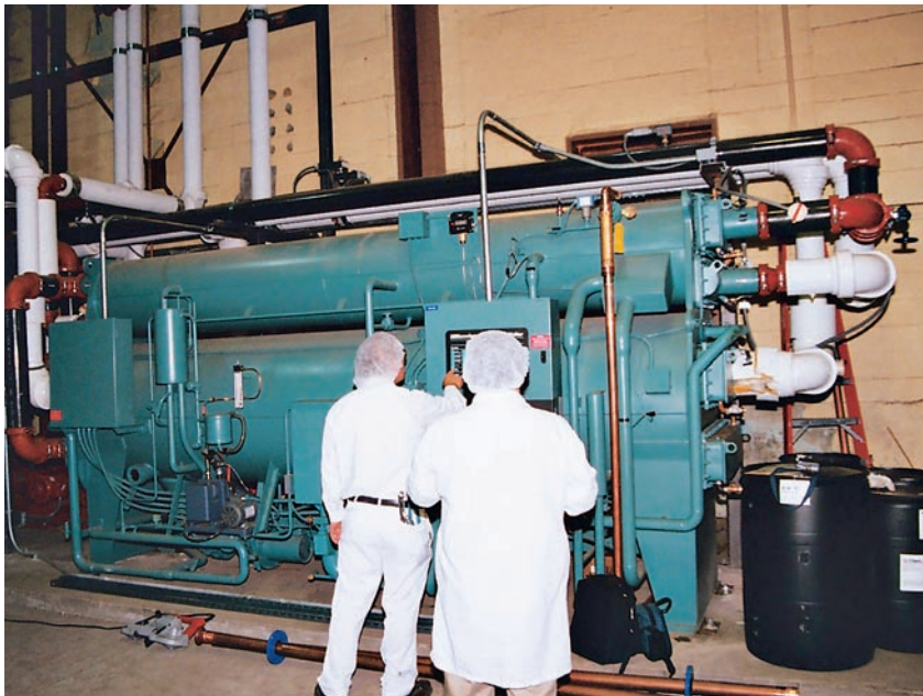
Absorption cooling provides process efficiencies, heat utilization for Ghirardelli Chocolate Company.
