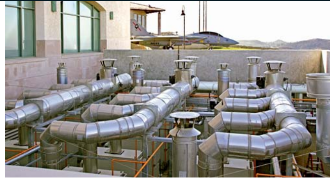
The equipment yard at the Ronald Reagan Library encompasses 16 Capstone microturbine units. Waste heat from 12 of the units supplies a Carrier absorption chiller. The other four supply building hot water.
