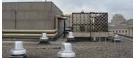
View of the microturbines from the roof of the Four Seasons Hotel.
