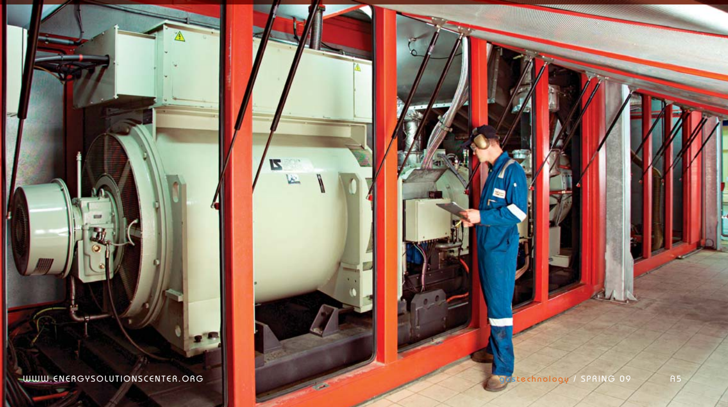
This 4.6 MW Mercury™ recuperative gas turbine by Solar Turbines provides hot water for a university hospital in France, and provides surplus electric energy to the regional grid. Photo courtesy Solar Turbines.
