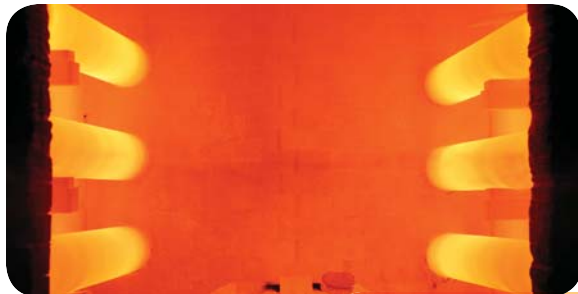
These six indirect-fired burners by Eclipse use recuperative firing for increased efficiency and reduced emissions. Photo courtesy Eclipse.
